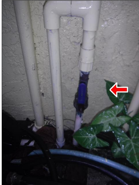
Main Water Shut Off Valve
