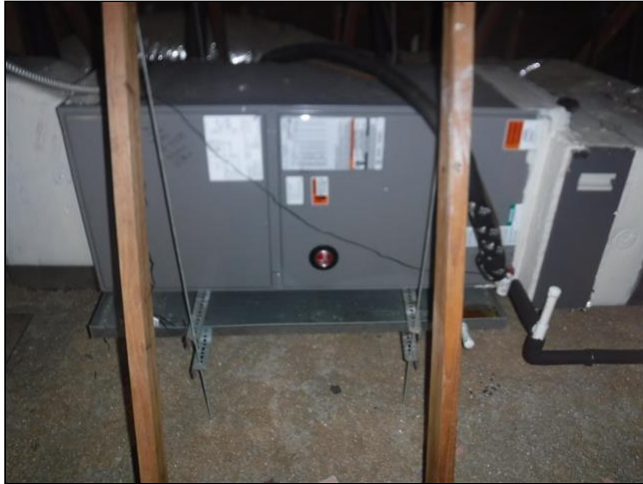
Attic Mounted Air Handler
