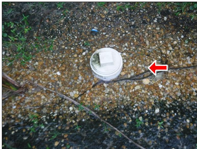
Main Plumbing Clean Outs
