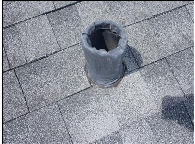
Plumbing Roof Vent
