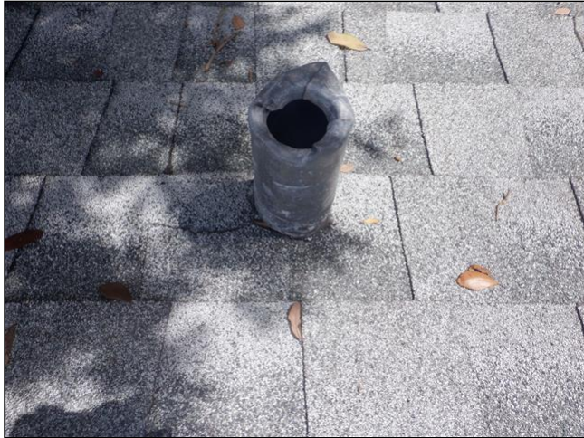
Plumbing Roof Vent
