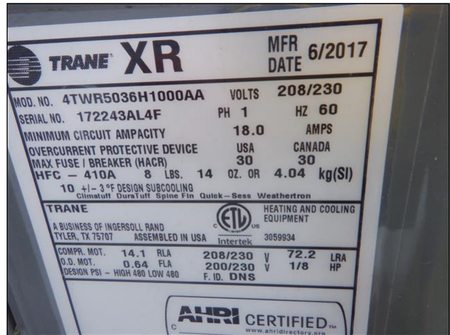
Condensing Unit ID Plate
